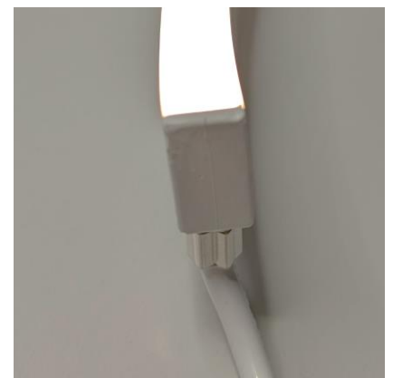
Rear Cable Entry (RE)
