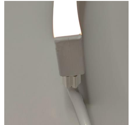
Rear Cable Entry (RE)
